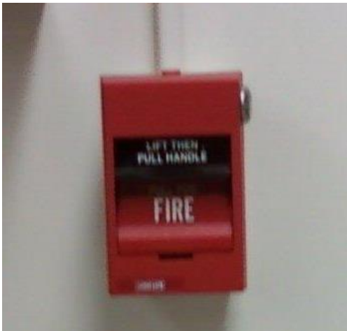
Figure 2: Example of building fire alarm
