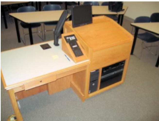
Extron Control Panel
